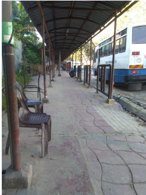
Figure 2. Improper bus stop design and conditions in Kota Kinabalu city
