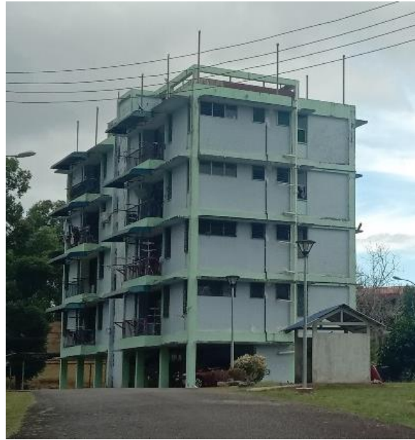
Figure 7. Typical buildings with weak and/or soft story
