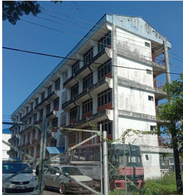
Figure 6. Typical buildings with beams do not align with columns
