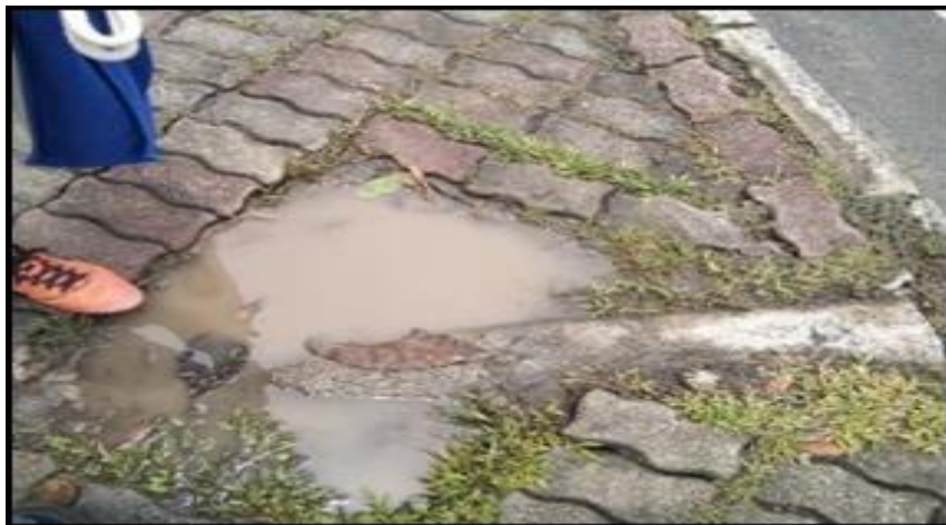
Figure 4. Pavement condition of walkway at Luyang.
